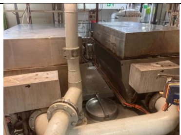
Photo #04 8/7/23 Image: IMG_0634 By: Dobrowski Description: MSD aeration tanks
