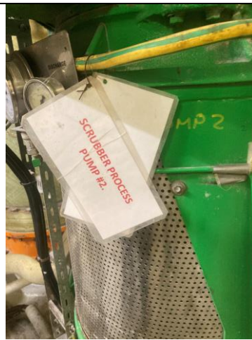
Photo #12 8/7/23 Image: IMG_0639 By: Dobrowski Description: EGCS pump
