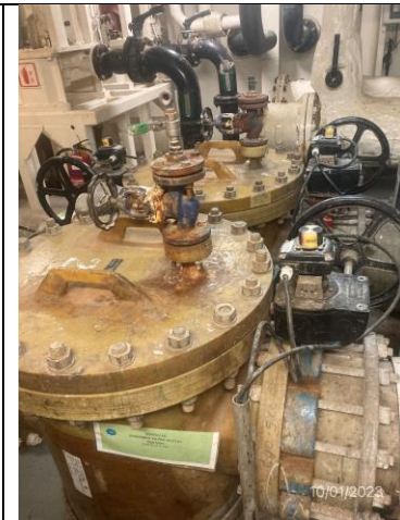
Photo #13 10/1/23 Image: IMG_E0791 By: Dobrowski Description: Wet Scrubber Filters
