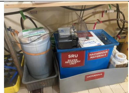
Photo #09 10/1/23 Image: IMG_E0804 By: Dobrowski Description: Silver Recovery Unit
