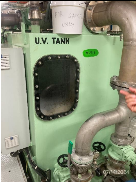
Photo # 17 Image: IMG_1833 Date: 7/14/2024 Taken by: Evan Dobrowski Description: Photo showing UV tank for MBR system.
