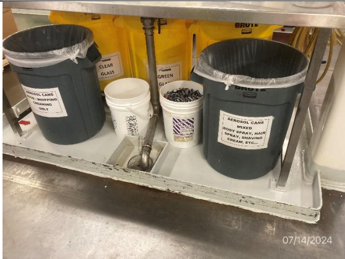
Photo # 7 Image: IMG_1808 Date: 7/14/2024 Taken by: Evan Dobrowski Description: Photo of sorting room battery and aerosol can storage.
