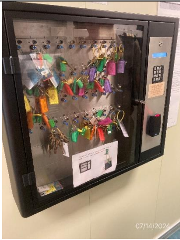
Photo # 13 Image: IMG_1822 Date: 7/14/2024 Taken by: Evan Dobrowski Description: Photo of keylock system.
