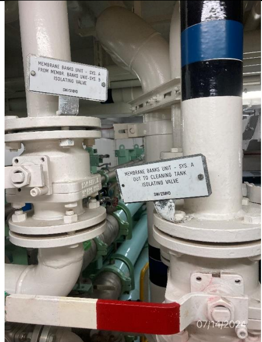
Photo # 16 Image: IMG_1828 Date: 7/14/2024 Taken by: Evan Dobrowski Description: Photo of Wartsila MBR isolation valves.
