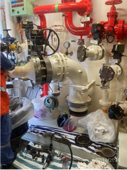
Photo # 5 Image: IMG_1803 Date: 7/14/2024 Taken by: Evan Dobrowski Description: Photo of fuel transfer room.
