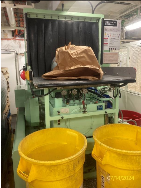
Photo # 11 Image: IMG_1813 Date: 7/14/2024 Taken by: Evan Dobrowski Description: Photo of incinerator shoot inside garbage sorting room.
