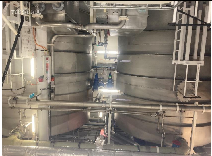
Photo # 4 Image: IMG_1520 Date: 5/13/2024 Taken by: Evan Dobrowski Description: wastewater holding tanks
