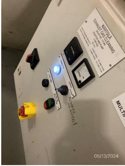
Photo # 13 Image: IMG_1529 Date: 5/13/2024 Taken by: Evan Dobrowski Description: EGCS pump controls
