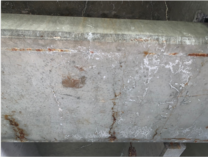
Photo 3: Cracks forming in the structural members of the top parking deck. Continued water intrusion causes the cracks to grow weakening the structure and will eventually cause failure of the structure.
