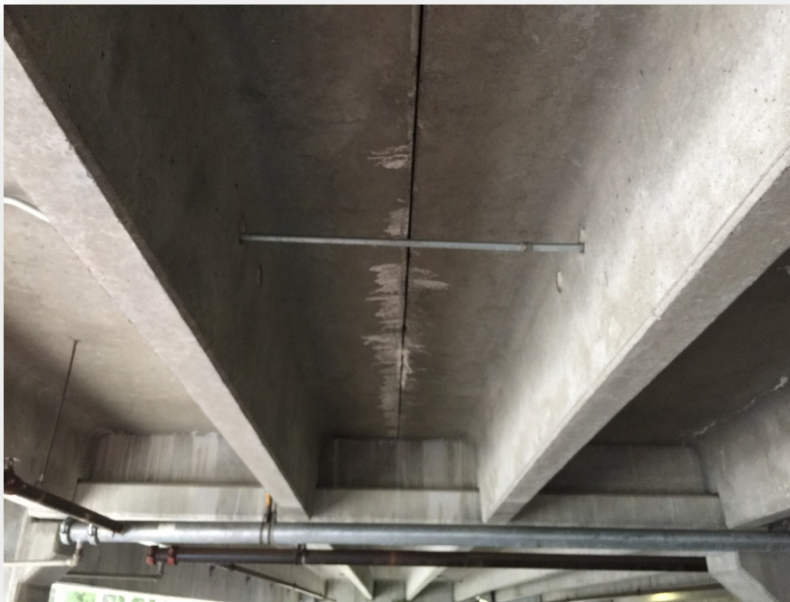
Photo 4: Joints between precast structural members showing water intrusion. Continued intrusion will cause failure of the joint.
