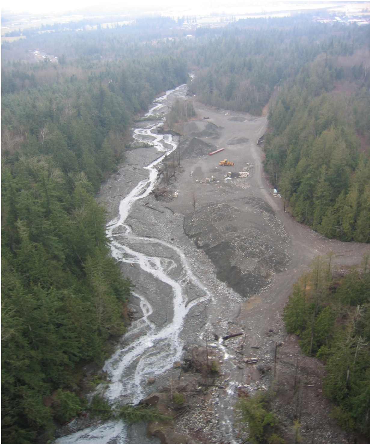
Figure 3: Great Western Lumber gravel removal operation along upper Swift Creek, 2009 (Source: Whatcom County)
