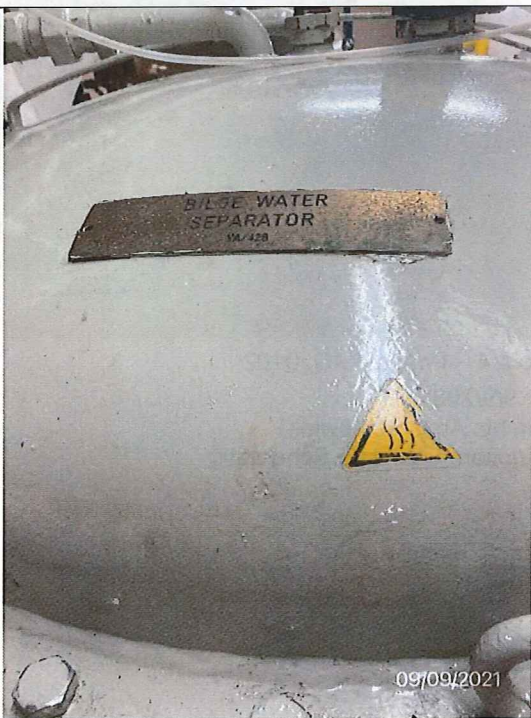
Photo # 7 Image: IMG_0248 Date: 9/9/2021 Taken by: Evan Dobrowski Description: Bilge – oily water separator (OWS)
