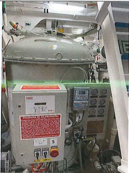
Photo # 17 Image: IMG_0123 Date: 9/9/2021 Taken by: Amy Jankowiak Description: Bilge – Oil Water Separator
