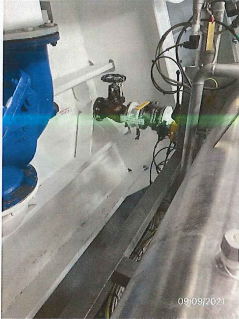
Photo # 9 Image: IMG_0241 Date: 9/9/2021 Taken by: Evan Dobrowski Description: Scanship – Overboard Discharge Port (Padlocked)
