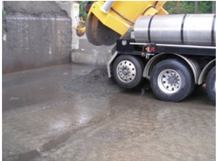
Vector truck dumping its load at a decant facility for proper waste handling.
