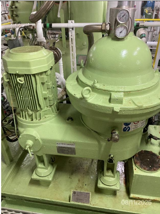
Photo # 7 Image: IMG_2951 Date: 8/11/2025 Taken by: Evan Dobrowski Description: Photo of bilge water separator.
