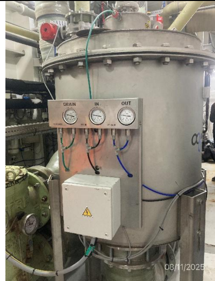
Photo # 20 Image: IMG_2974 Date: 8/11/2025 Taken by: Evan Dobrowski Description: Photo showing filtration for EGCS.
