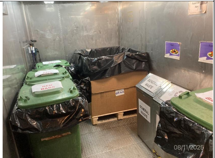
Photo # 12 Image: IMG_2967 Date: 8/11/2025 Taken by: Evan Dobrowski Description: Photo of hazardous waste storage area.
