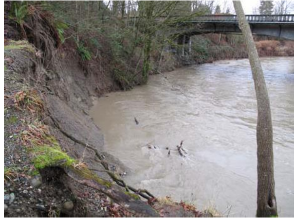
Bank erosion south of 2 nd St/ 92 nd St bridge
