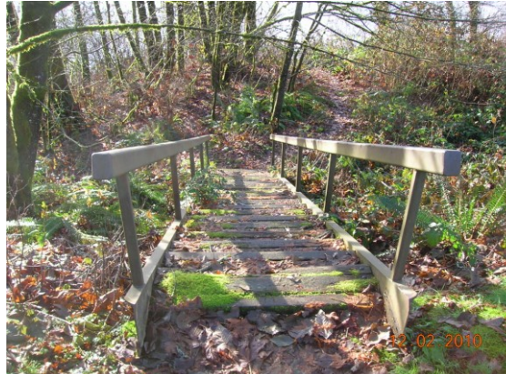
(Photo 4: (Segment 4) View south showing dilapidated stairway access to Skagit River to be removed by WSDOT.
