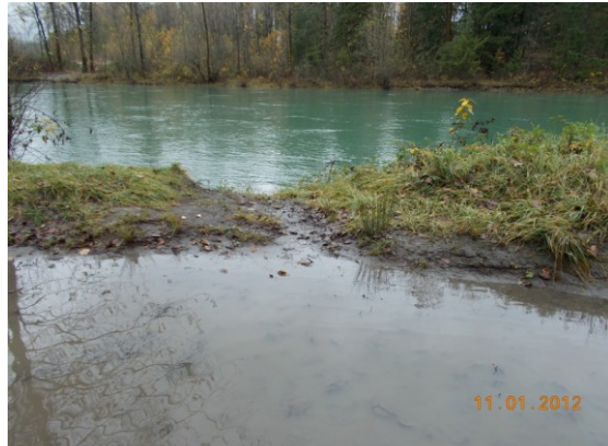
Photo 2: (Segment 3) View west showing stormwater discharging to Baker River from access road shown in Photo 1.
