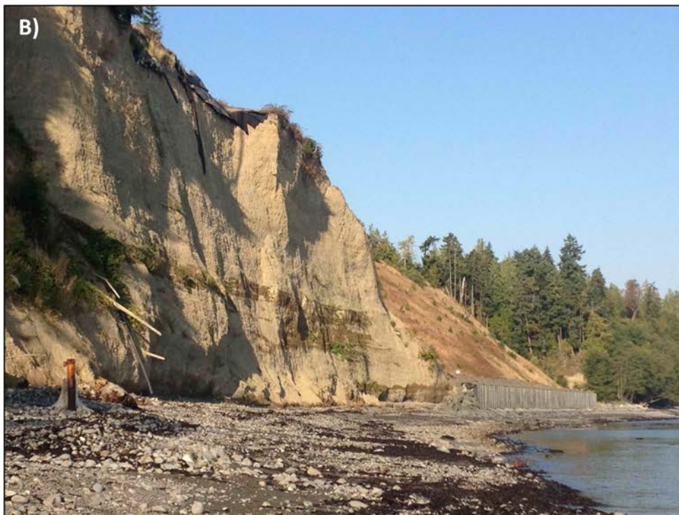
Figure 1. A) Bluff-top homes threatened by receding bluffs, Dungeness drift cell. B) Seawall installed at bluff toe to protect Port Angeles City Landfill from bluff retreat, Elwha drift cell.
