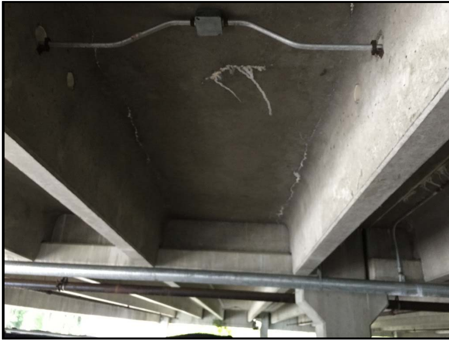
Photo 3: Cracks forming in the structural members of the top parking deck. Continued water intrusion causes the cracks to grow weakening the structure and will eventually cause failure of the structure.
