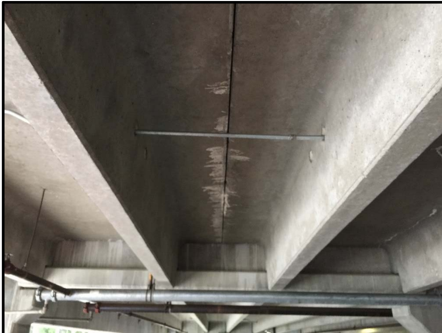
Photo 4: Joints between precast structural members showing water intrusion. Continued intrusion will cause failure of the joint.
