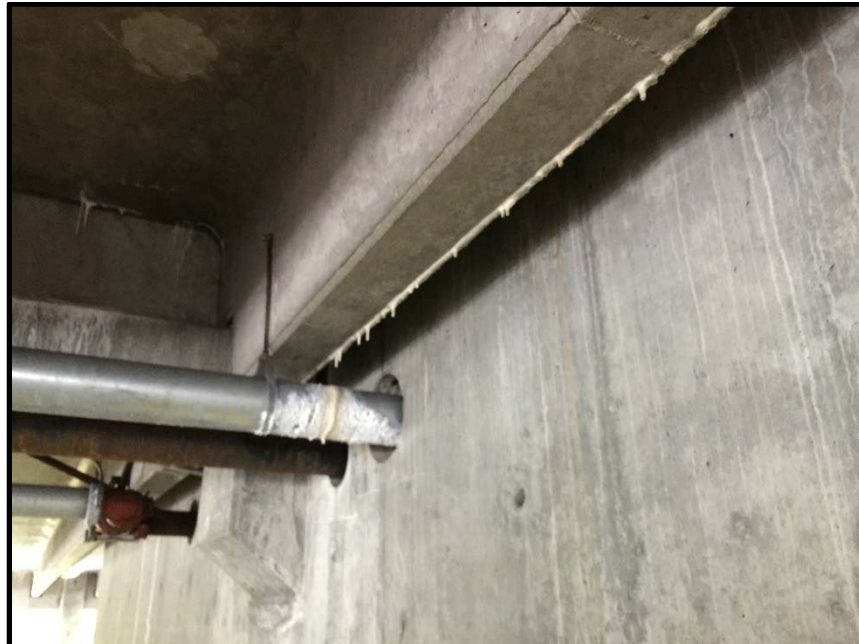
Photo 1: Water seeping through the concrete upper parking deck washing the minerals out of the structural concrete elements weakening the overall structure.
