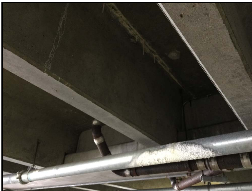
Photo 2: The bright colored pipe is part of the fire sprinkler system and was replaced recently due to corrosion from the leaks. Also cracks in the structural elements of the garage are forming and growing due to the water intrusion.
