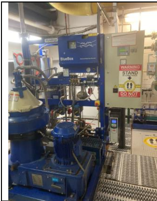
Photo #05 5/8/23 Image: IMG_204 By: Dobrowski Description: OWS oil content meter
