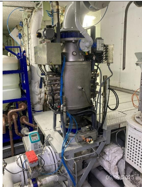
Photo # 4 Image: IMG_3106 Date: 9/9/2025 Taken by: Evan Dobrowski Description: Photo of UV filter component for the oily bilge filtration system.
