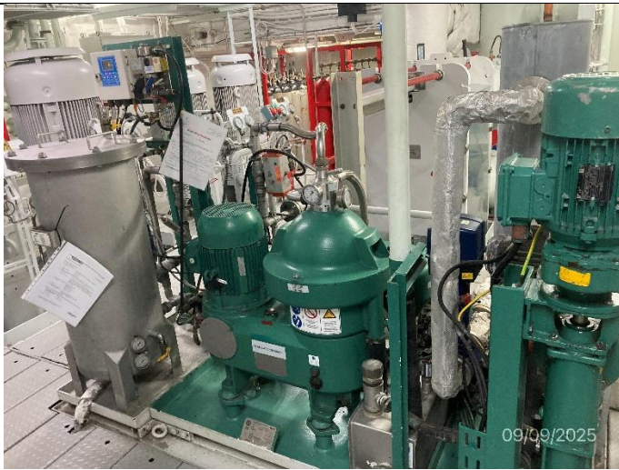
Photo # 3 Image: IMG_3103 Date: 9/9/2025 Taken by: Evan Dobrowski Description: Photo Centrifugal Oil Water Separator filter.
