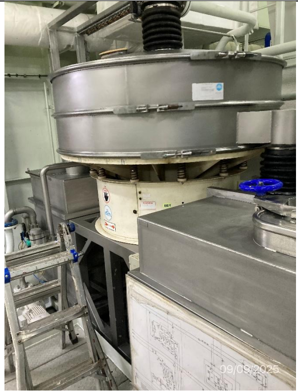
Photo # 2 Image: IMG_3097 Date: 9/9/2025 Taken by: Evan Dobrowski Description: Photo of MBR treatment system mixing tank
