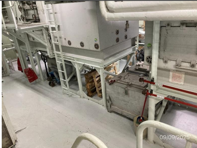
Photo # 5 Image: IMG_3108 Date: 9/9/2025 Taken by: Evan Dobrowski Description: Photo of incinerator room.
