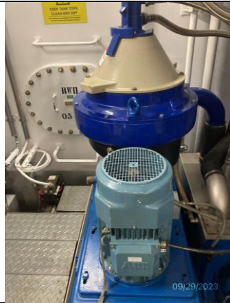
Photo #05 9/29/23 Image: IMG_E739 By: Dobrowski Description: OWS oil treatment
