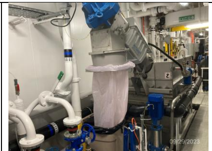
Photo #13 9/29/23 Image: IMG_0724 By: Dobrowski Description: SCR filter
