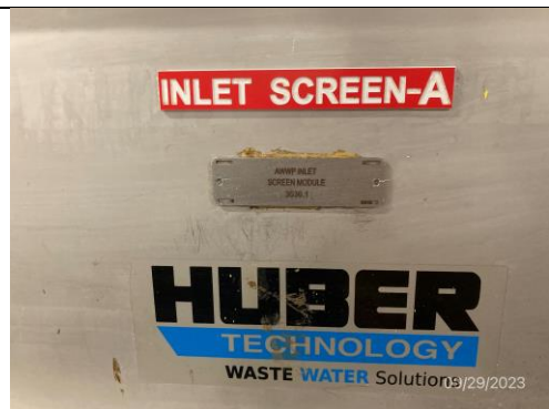
Photo #04 9/29/23 Image: IMG_E0725 By: Dobrowski Description: MSD inlet screen tank
