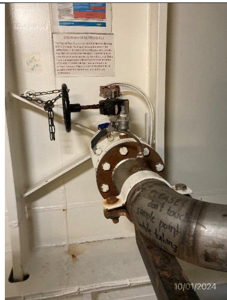
Photo # 12 Image: IMG_2089 Date: 10/1/2024 Taken by: Evan Dobrowski Description: Photo of blackwater overboard discharge shut and locked manually.
