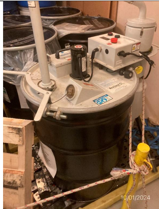
Photo # 16 Image: IMG_2108 Date: 10/1/2024 Taken by: Evan Dobrowski Description: Photo of Bulb Crusher.
