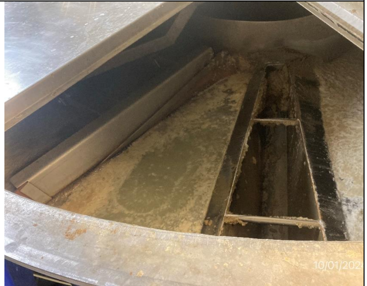
Photo # 10 Image: IMG_2084 Date: 10/1/2024 Taken by: Evan Dobrowski Description: Photo of interior of flocculation tank B.
