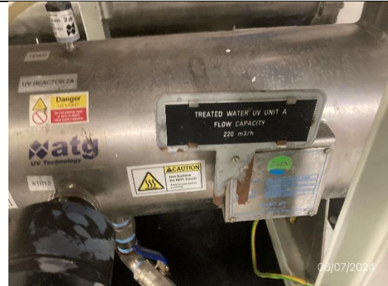
Photo # 32 Image: IMG_1703 Date: 6/7/2024 Taken by: Evan Dobrowski Description: Sewage treatment UV filter unit.
