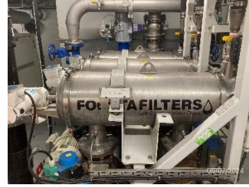
Photo # 30 Image: IMG_1701 Date: 6/7/2024 Taken by: Evan Dobrowski Description: Sewage treatment filters
