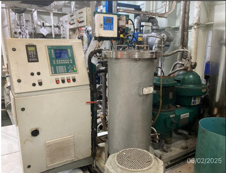
Photo # 8 Image: IMG_2811 Date: 6/2/2025 Taken by: Evan Dobrowski Description: Photo of centrifugal oil water separator.
