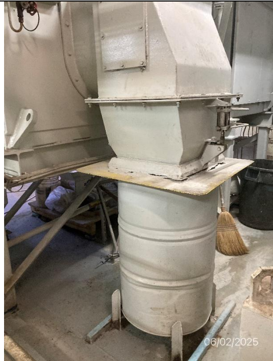
Photo # 10 Image: IMG_2813 Date: 6/2/2025 Taken by: Evan Dobrowski Description: Photo of incinerator ash chute.
