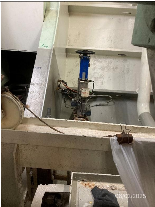
Photo # 6 Image: IMG_2807 Date: 6/2/2025 Taken by: Evan Dobrowski Description: Photo of blackwater MBR discharge valve with padlock.
