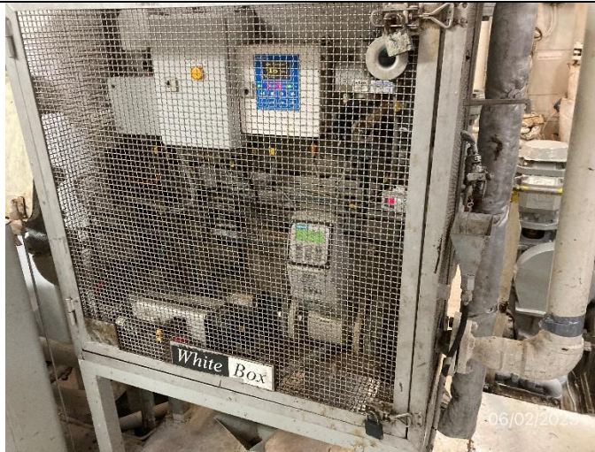
Photo # 9 Image: IMG_2812 Date: 6/2/2025 Taken by: Evan Dobrowski Description: Photo of Marinfloc Whitebox unit double locked.
