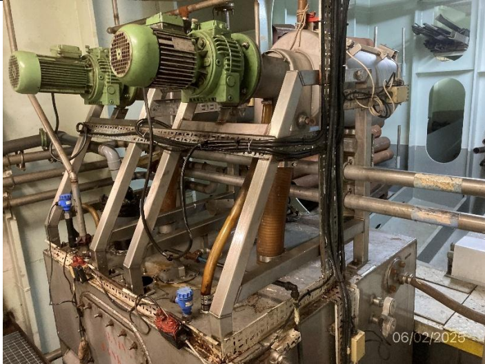
Photo # 4 Image: IMG_2804 Date: 6/2/2025 Taken by: Evan Dobrowski Description: Photo of MBR dewatering first stage system.
